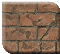
FIRE CRACKED BRICK
