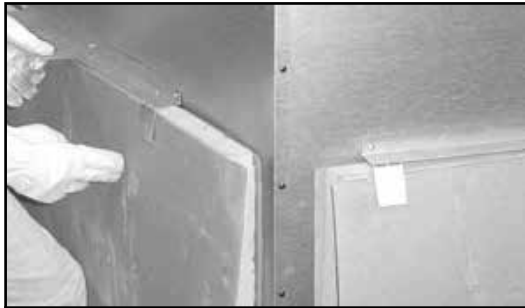
Figure 3.5 Unpack Back Refractory
